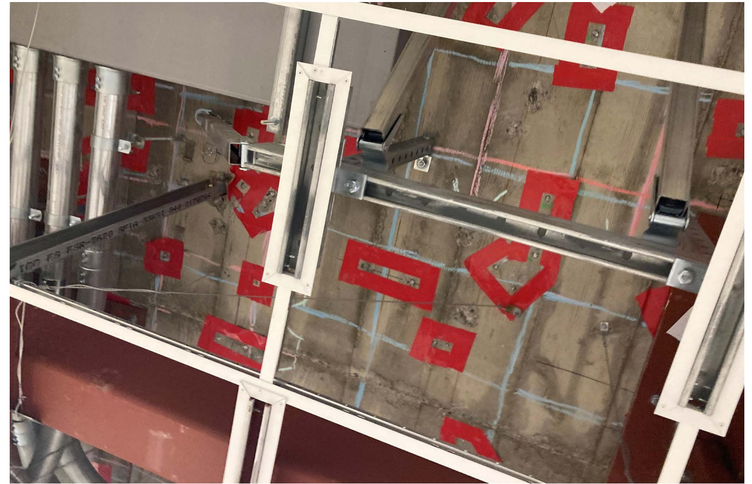
In this image, tape around each existing anchor defines how far away a new anchor would need to be placed to move equipment, as well as lines showing the rebar that must be avoided.
